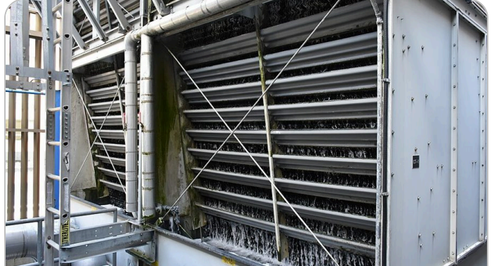
Fill media inside a cooling tower — where water film meets the air
