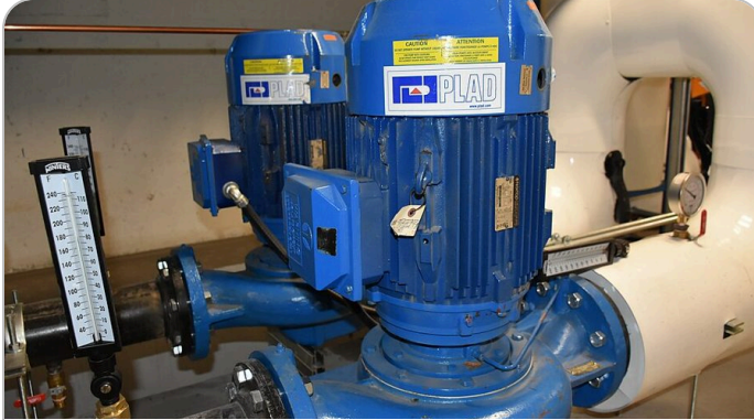
Close-coupled centrifugal pumps with pressure gauges on suction and discharge
