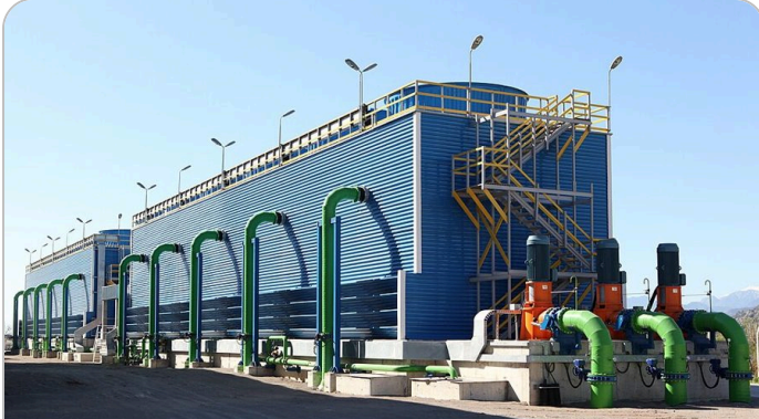
Induced-draft cooling tower cells with fans on top
