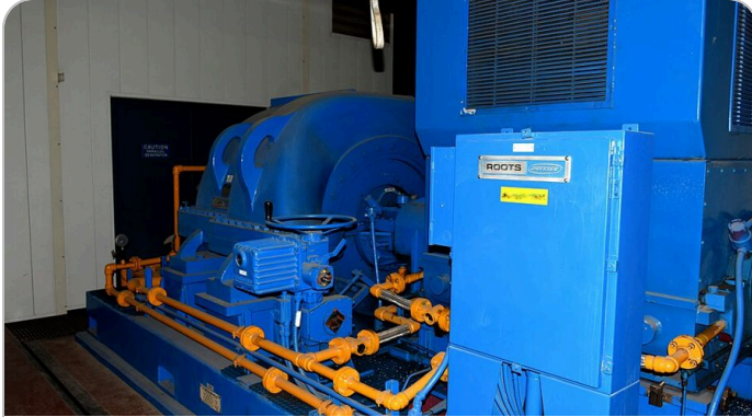
Industrial centrifugal fan on its motor base
